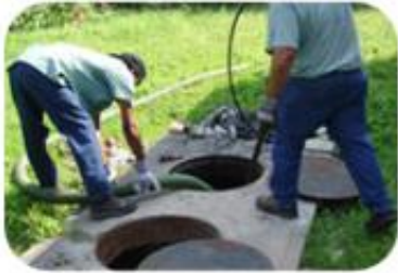
Gravity Grease Interceptor (GGI) - outside, concrete
