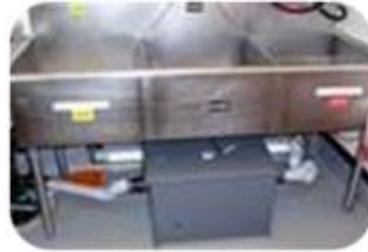
Hydro-mechanical Grease Interceptor (HGI) - In floor or under a sink
