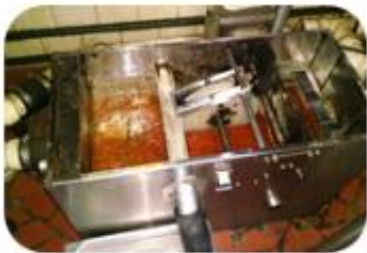
Automatic Grease Removal Device - plugged in
